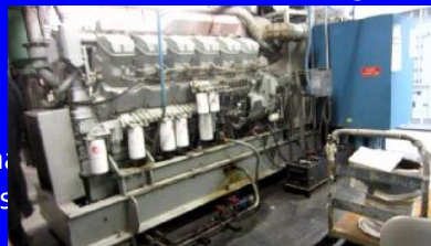
This is the Actual Coney Island Hospital Generator that was salvaged
